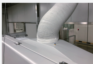
Exhaust Hood and Pipe
